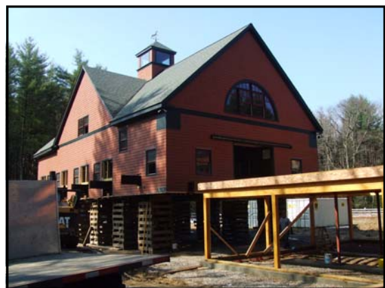
The Barn at 190 Concord Road being moved off the land that is protected by a CR
